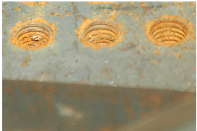
Figure 7. Unacceptable Rust in Coupler Threads
