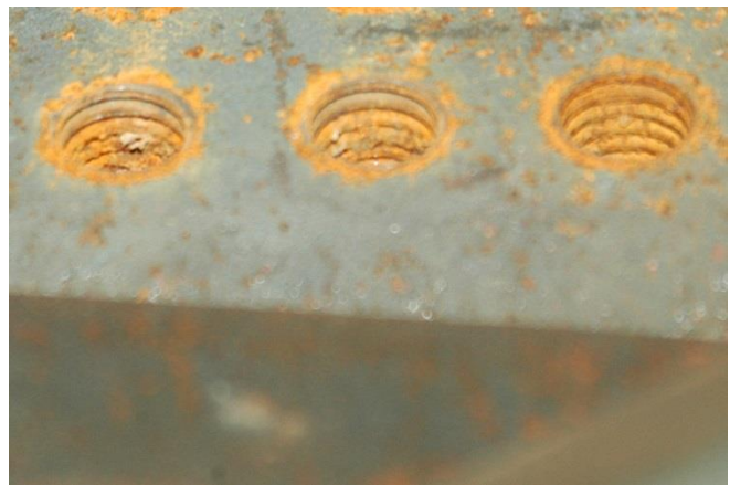
Figure 6. Unacceptable Rust in Coupler Threads
