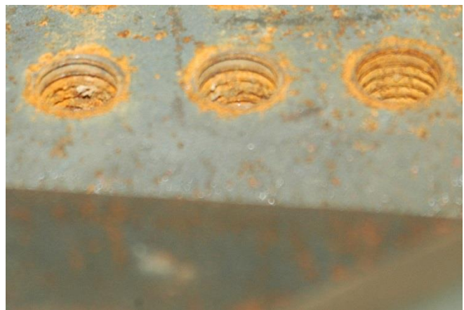
Figure 6. Unacceptable Rust in Coupler Threads
