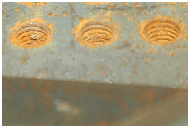
Figure 6. Unacceptable Rust in Coupler Threads
