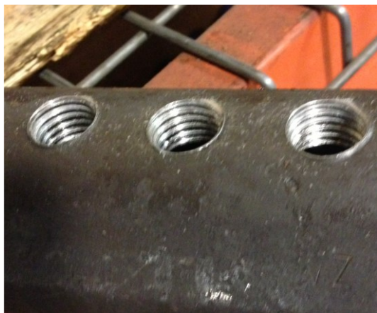
Figure 5. Clean Acceptable Coupler
