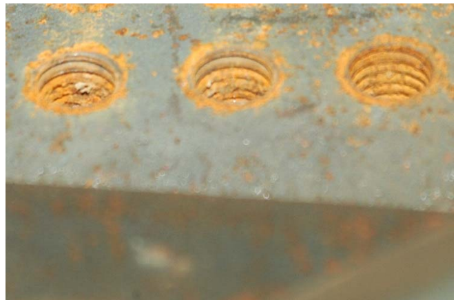
Figure 6. Unacceptable Rust in Coupler Threads
