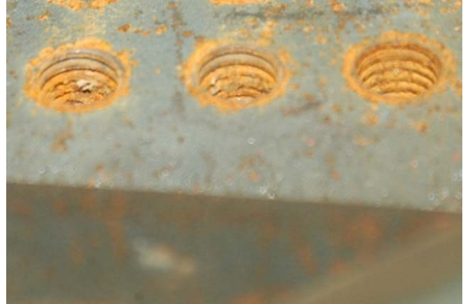
Figure 5. Unacceptable Rust in Coupler Threads
