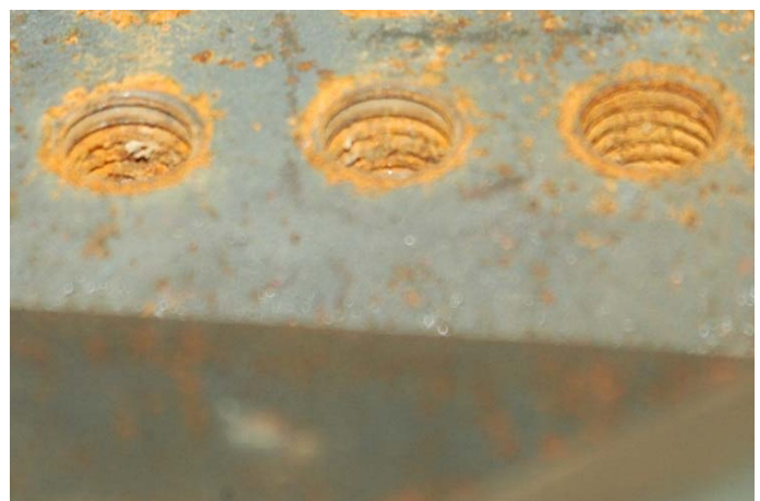
Figure 6. Unacceptable Rust in Coupler Threads
