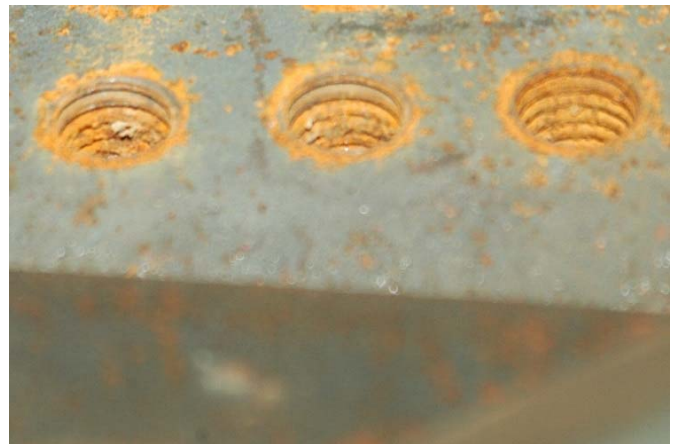
Figure 6. Unacceptable Rust in Coupler Threads
